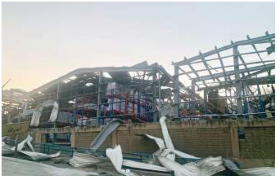
The impact of 2020 Beirut explosion! The NET destroyed warehouses in Beirut Port
