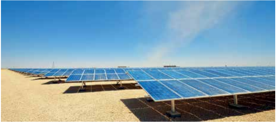
Saudi Arabia's renewable push: King Abdullah Petroleum Studies and Research Center (KAPSARC) solar power plant (image credit: Phoenix Solar AG)
